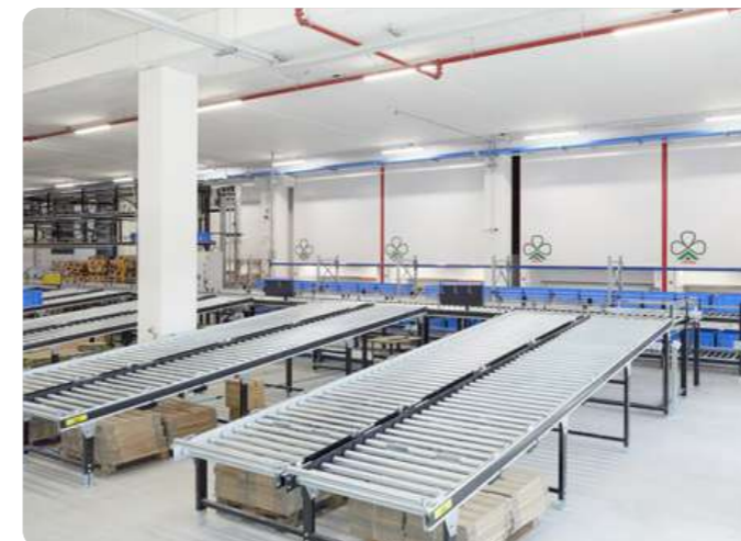
CONVEYOR BELTS AND ROLLER UNITS
